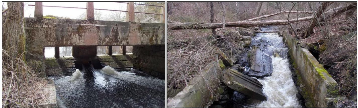
Figure 3: Horseshoe Mill Dam Spillway and Bridge from Downstream Side (left) and Former Mill Race (right)
