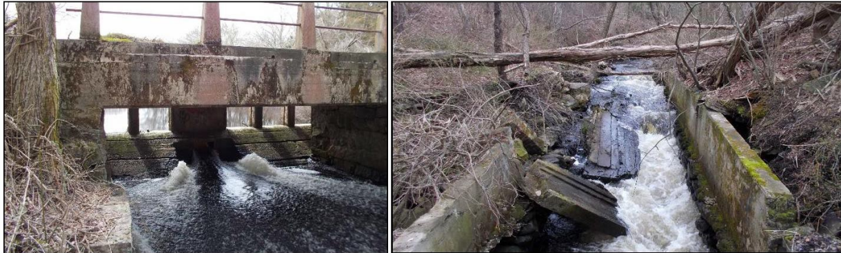
Figure 3. Horseshoe Mill Dam Spillway and Bridge from Downstream Side (left) and Former Mill Race (right)
